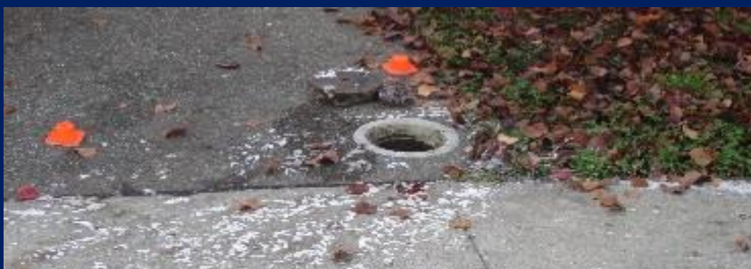
Overflow from clean out
