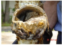
Grease Clogged Pipe
