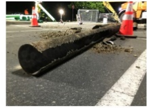
FOG Related Deterioration
