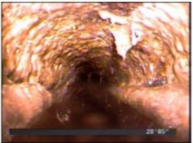
Grease Coated Pipe
