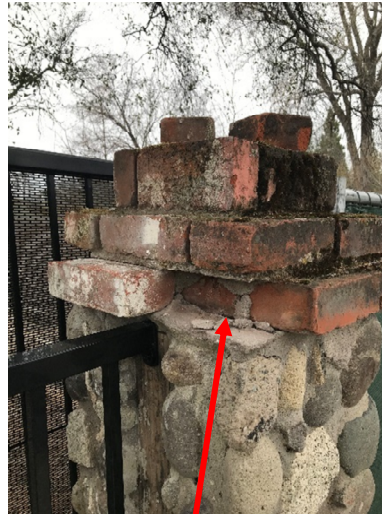
Replace missing brick and mortar.
