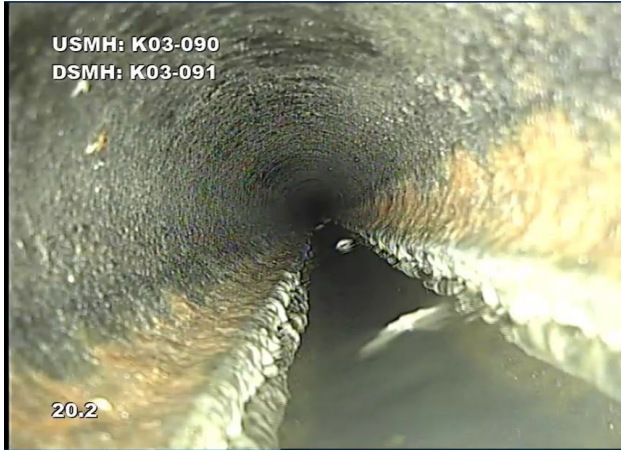
Photo 1 - 02/13/2023 – Excessive grease accumulation documented in public sewer system that serves Lucille’s Smokehouse BBQ via CCTV.
