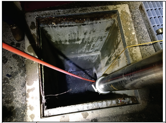
Date Vacuum tube from SPMUD vacuum truck removing SSO contents from storm drain inlet. 3/22/18
