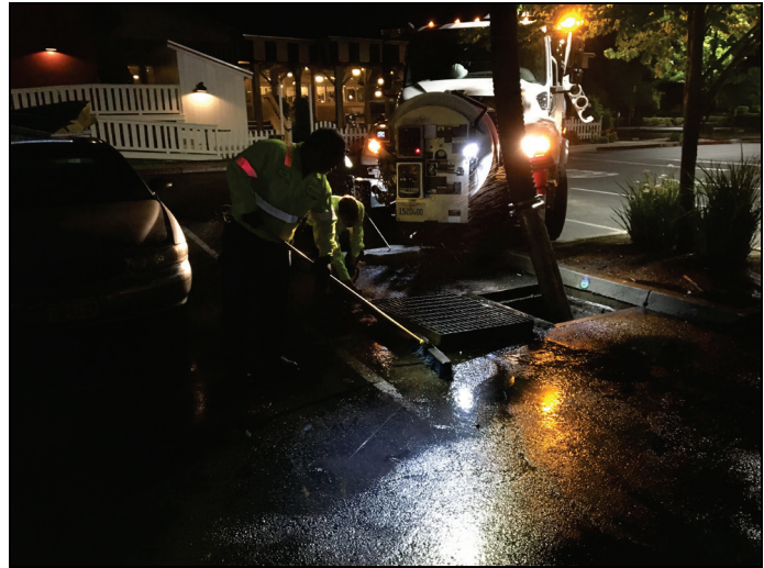
Date SSO was cleaned up by SPMUD crew. Contents were vacuumed out of City of Rocklin storm drains. 5/17/19
