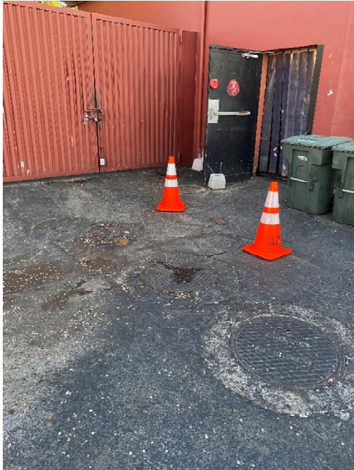
Photo 9 - 03/20/2023 - Grease staining on AC pavement around cleanouts and grease interceptor.
