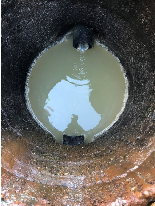
Photo 5 - 03/20/2023 - District staff document condition of sampling box prior to taking effluent samples.
