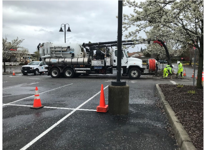
Photo 3 - 03/15/2023 – District crews hydro excavate in Lucille’s drive aisle/parking lot to retrieve stuck cleaning nozzle.
