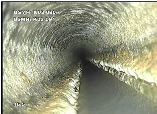
Photo 2 - 02/13/2023 - Excessive grease accumulation documented in public sewer system that serves Lucille’s Smokehouse BBQ via CCTV.
