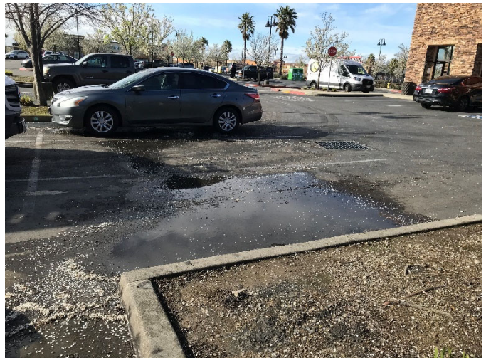
Photo 12 - 03/20/2023 - Grease staining leading to storm drain inlet.
