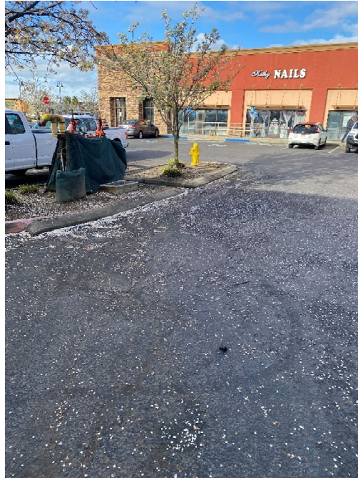
Photo 11 - 03/20/2023 - Grease staining through parking lot, surface area is slick/slippery.
