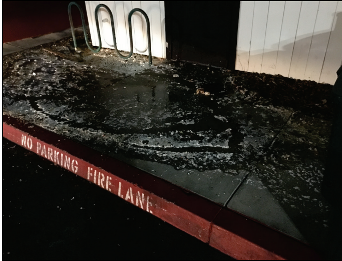
Date Sanitary sewer overflow (SSO) from private two-way cleanout at west backdoor of Lucille’s BBQ. 5/17/19
