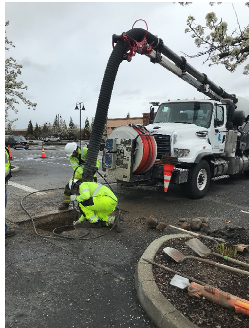
Photo 4 - 03/15/2023 – District crews hydro excavate in Lucille’s drive aisle/parking lot to retrieve stuck cleaning nozzle.
