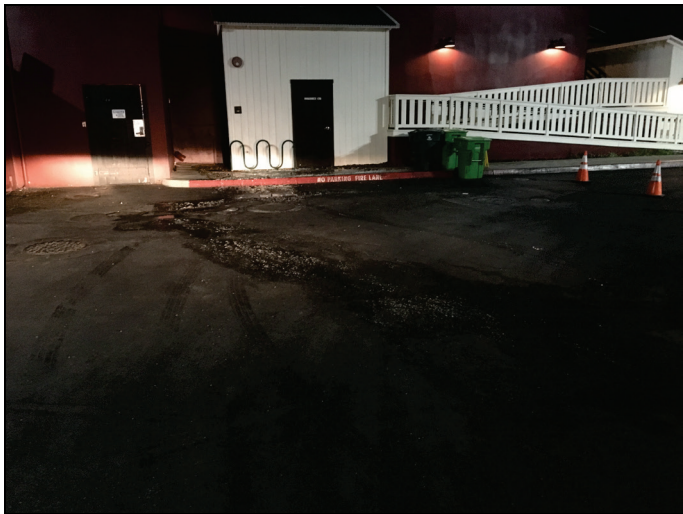
Date SSO drained from west backdoor through parking lot. 5/17/19
