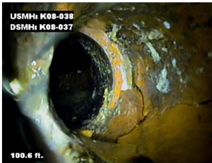
Spiral fracture at the wye at 3185 Midas Avenue.
