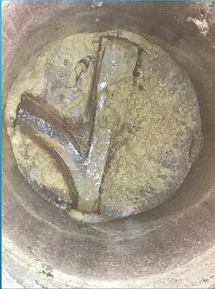
Heavy solids discharge lead to a blockage resulting in a sewer overflow
