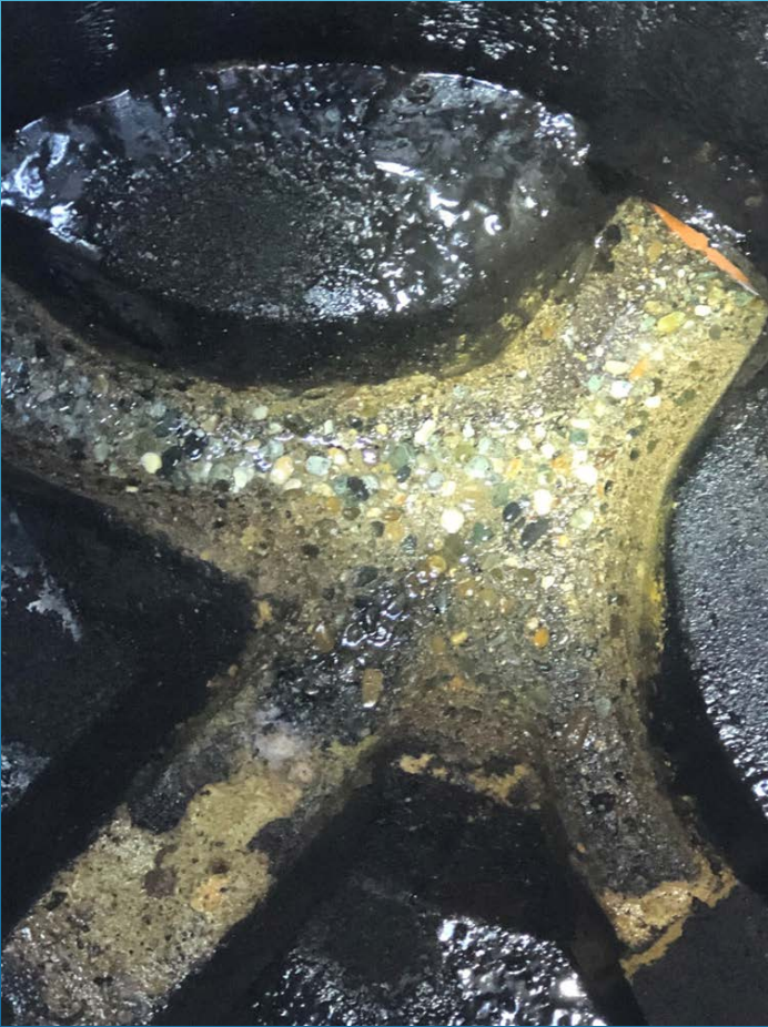
Corrosion in manhole channels lead to exposed aggregate
